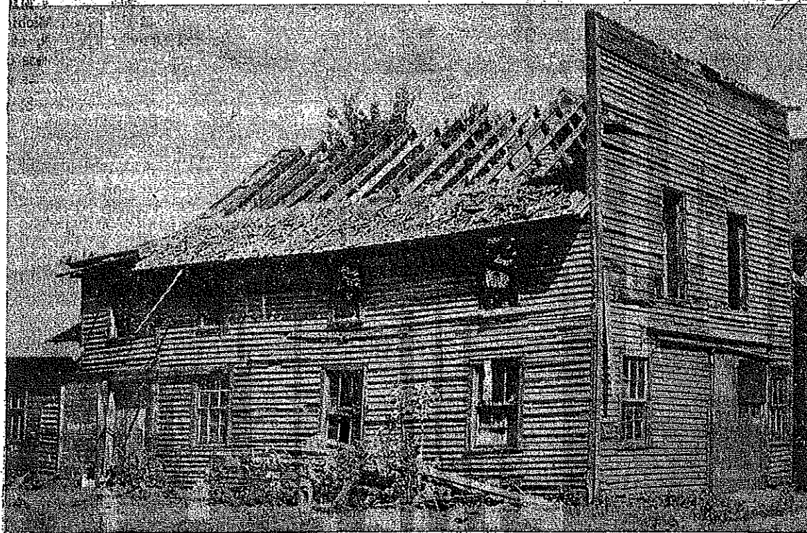
HISTORIC monument to Petoskey's early horse and buggy days is starting to disappear. The old McDermott blacksmith shop is now being torn down by two Petoskey workers to make way for more modern improvements. The building, erected before the turn of the century, was part of the old trading area for farmers who made regular visits to the village smithy for wagon repairs and new shoes for their teams. The property is owned by Mrs. Alma Barnes, last survivor of the McDermott-Schofield families. The rear of the building, a residence in the early days, will be saved for future use. (News-Review photo by Fred Lovelace)
